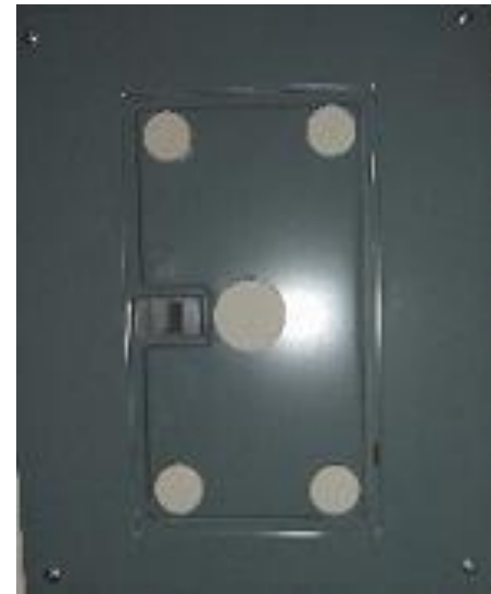
Fuse Box Protection
